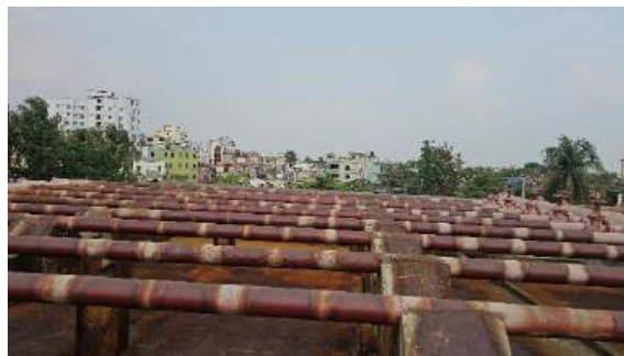
Photo 3: Inlet of GWTP at CuCC
