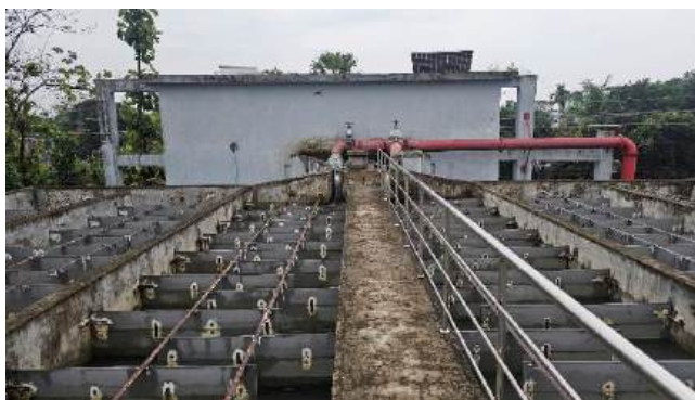
Clarifier tanks of SWTP
