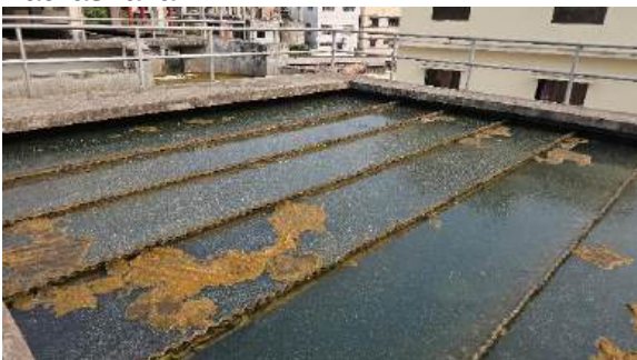
Photo 3: GWTP at CuCC
