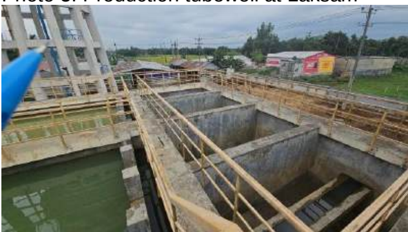
Photo 7: Groundwater treatment plant in Laksam Paurashava.
