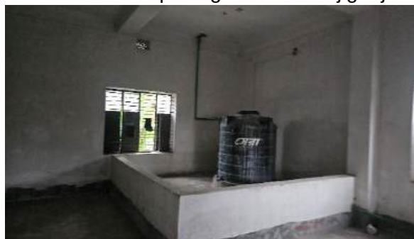
Photo 8: Chlorine dosing tank at Chandpur Paurashava.
