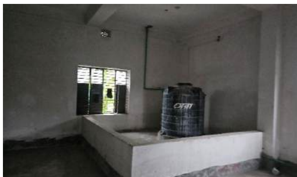
Photo 14: Chlotine dosing tank at SWTP Puranbazar, Chandpur
