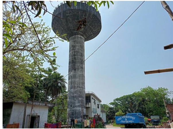
Photo 12: Water Reservoir at Natore
