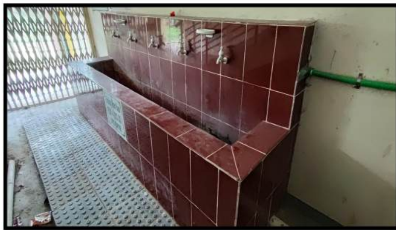
Fig. 13 Five Outlet Water Collection Basin
