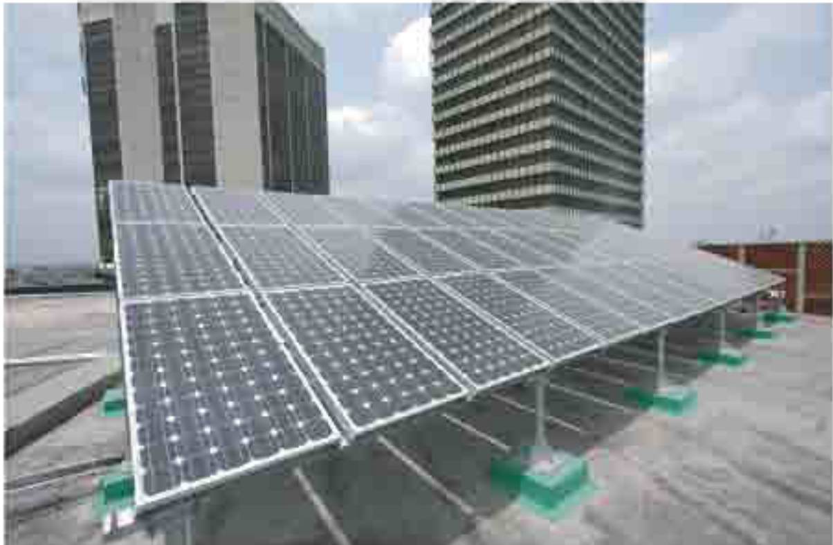
Solar panel on the roof-top of commercial buildings can be a solution to GHG emission
