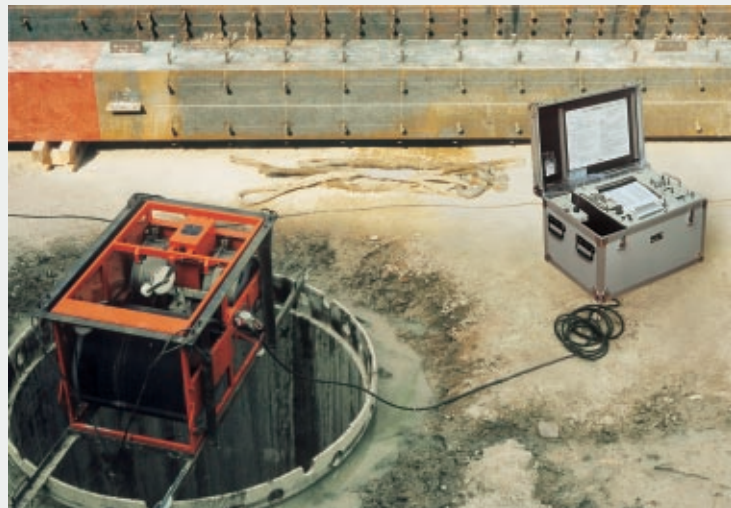
The winch unit and recorder unit on site
