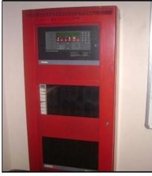
Fire Alarm Panel
