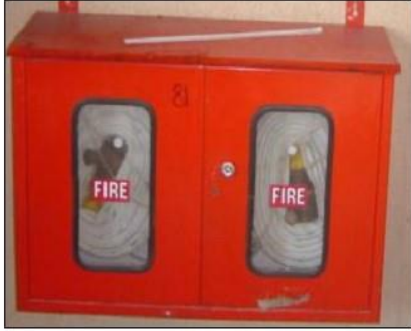
Water Hoses & inlet
