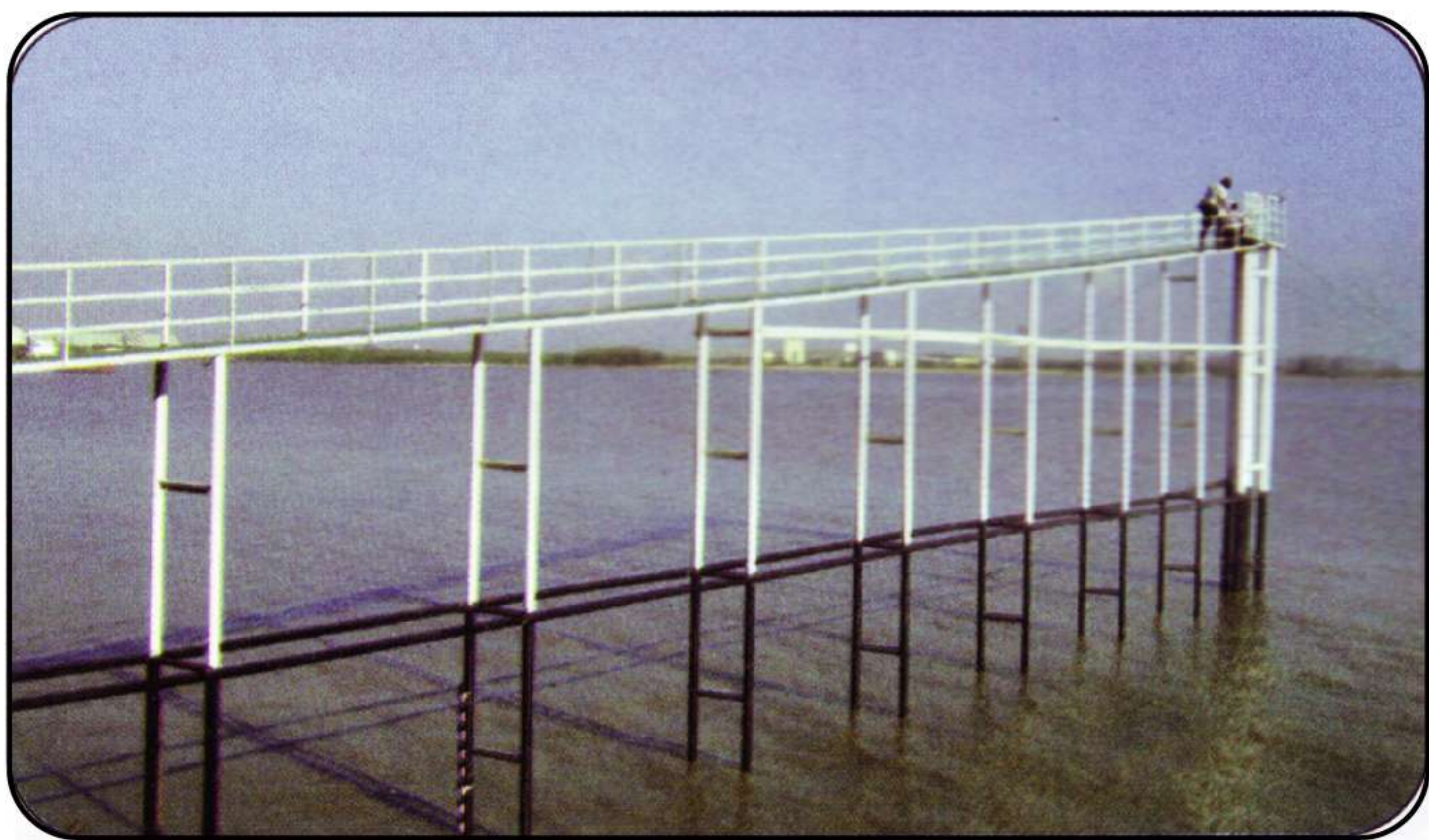
Auto Tide Gauge Station at Khal 18
