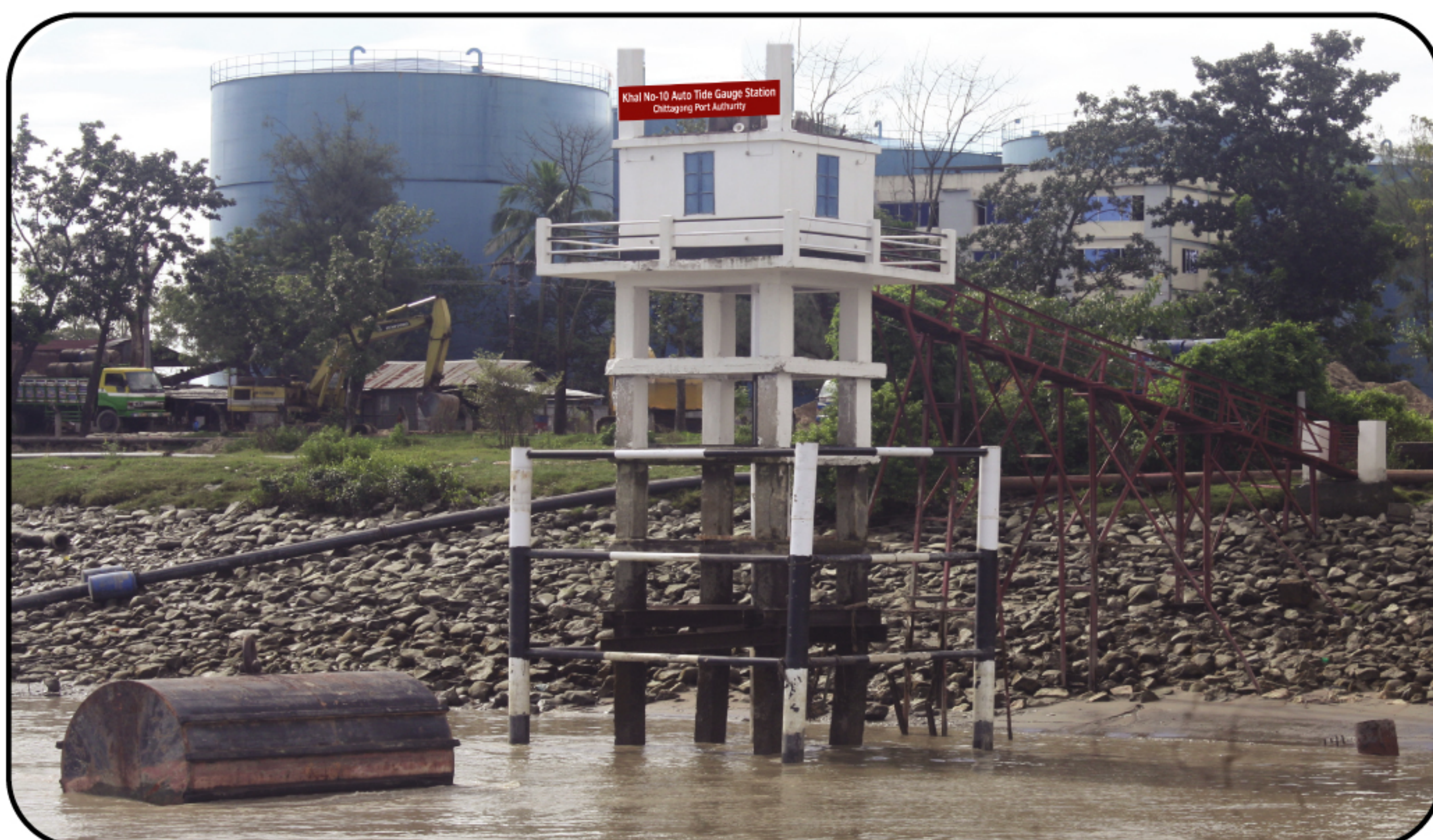
Auto Tide Gauge Station at Khal No-10
