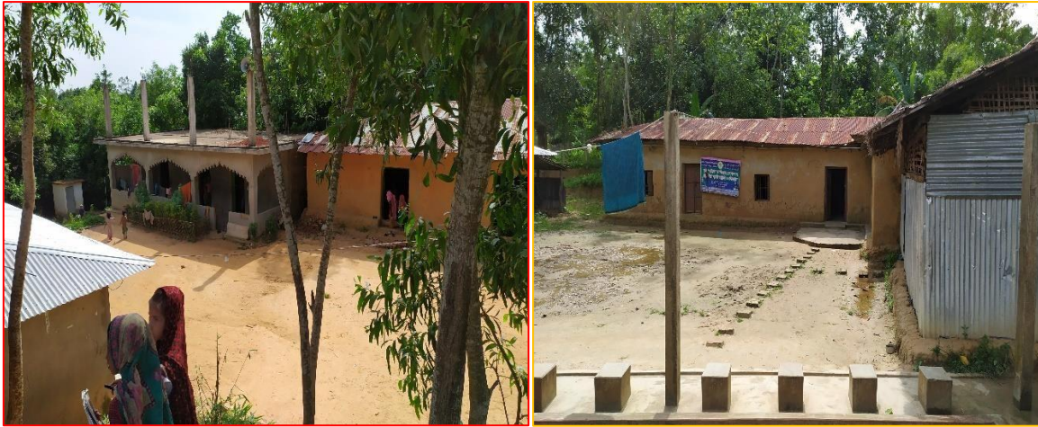
Figure 5: Madrasayе Saiyedena in ward no 3 (left) which was damaged by cyclone SIDR; Mohammedia Talimul Quran madrasa in ward no 1 (right) which is prone to flash flood.
