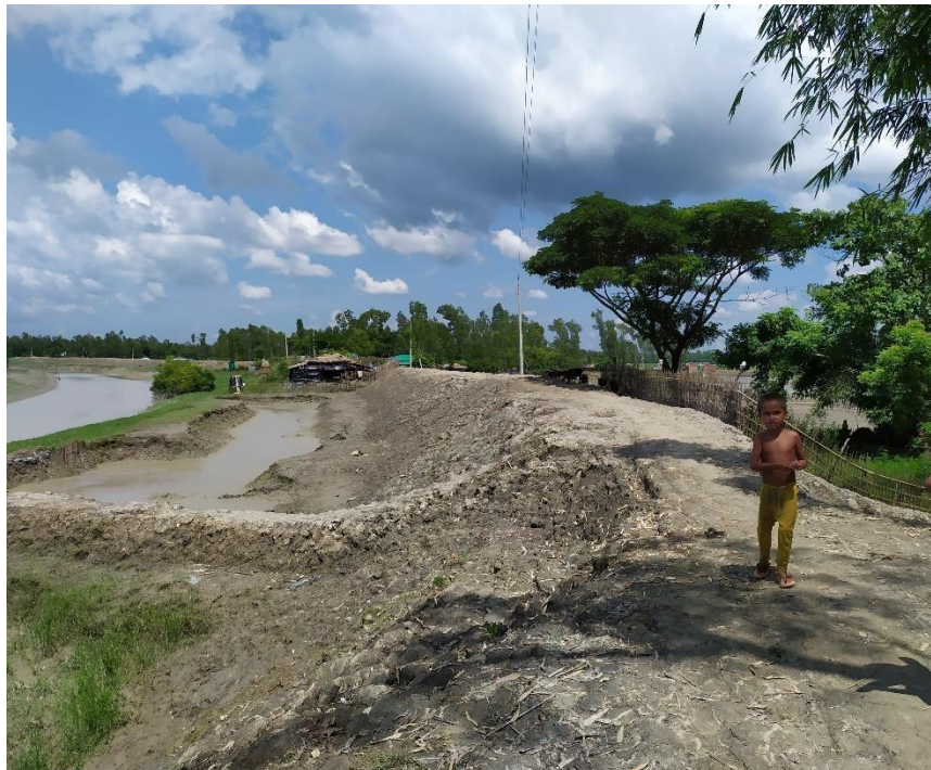
Figure 2: WAPDA embankment in ward no 6, prone to coastal flooding.
