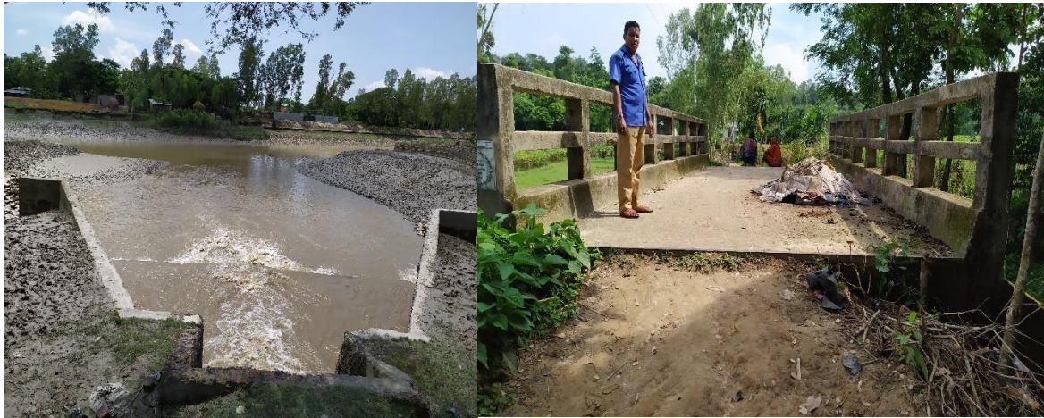
Figure 7: Kotapara in ward no 6 (left) causes flooding because of sedimentation; bridge situated in ward no1, prone to flooding (right).
