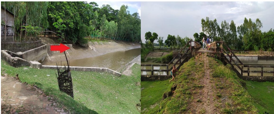
Figure 4: Broken guide wall beside Nonaichori canal in ward no 2 (left), rubber dam in ward no 6 which needs attention (right).
