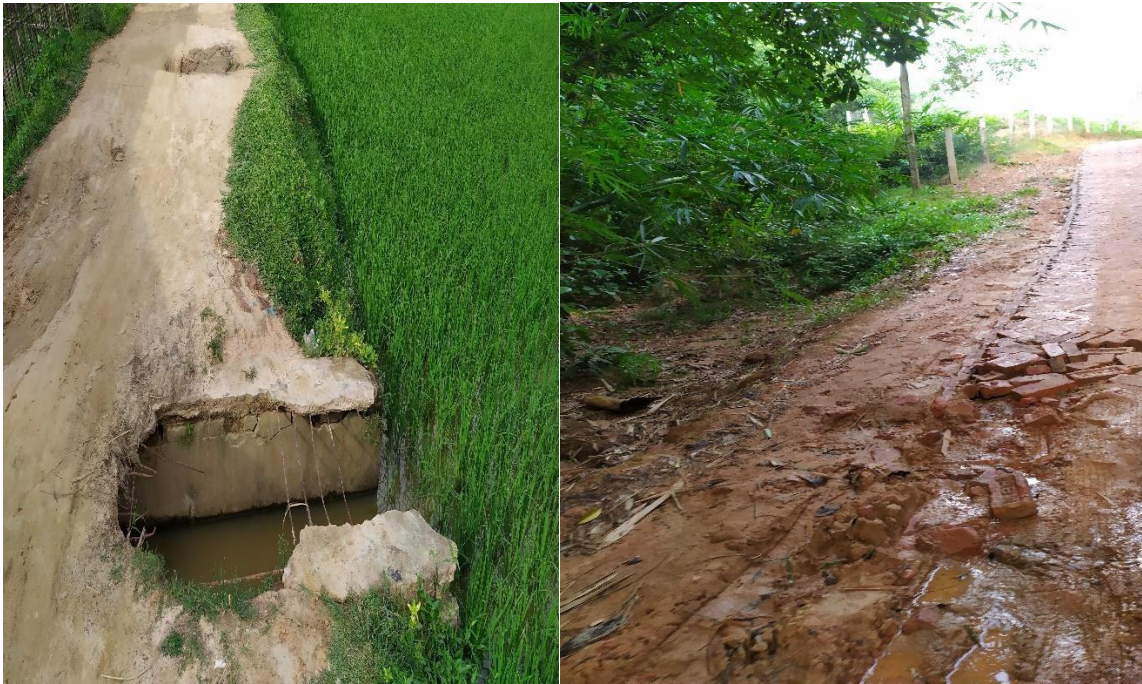
Figure 1: Jonaimura road in ward no 5 (left), another vulnerable road in ward no 5 (right); both are prone to flooding.
