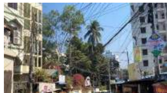
Figure 8-12: Tangled Power and Internet Cables.
