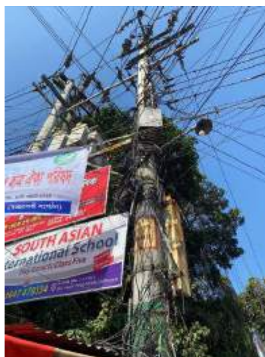
Figure 8-10: Cluster of Wires
