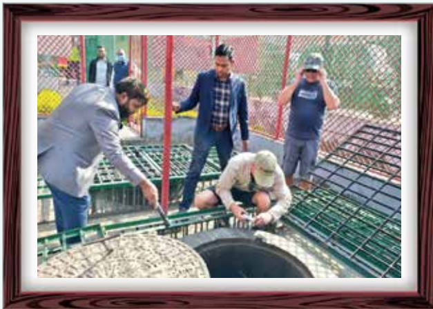
A moment of ongoing survey at Cox's Bazar Beachmahole area for installation of SMW-6 Submarine Cable
