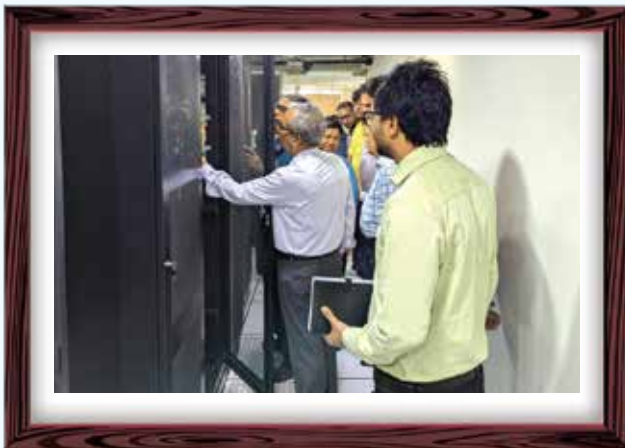
Managing Director of BSCPLC visiting the IIG Network Operation Center.
