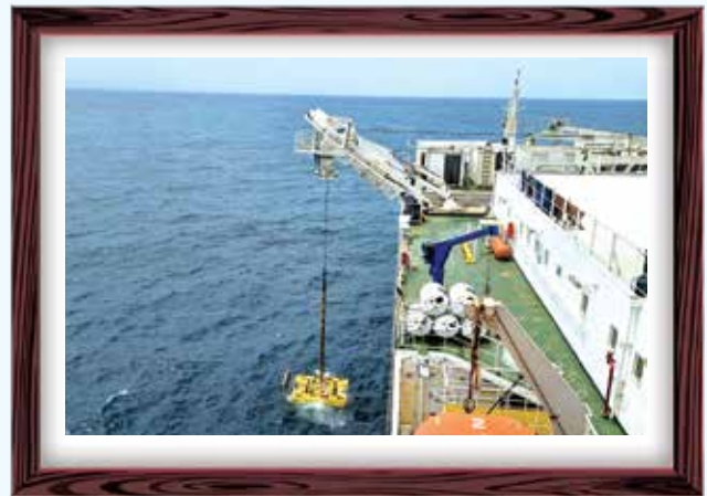
Installation of Cox's bazar branch of SMW-6 submarine cable system at deep sea.
