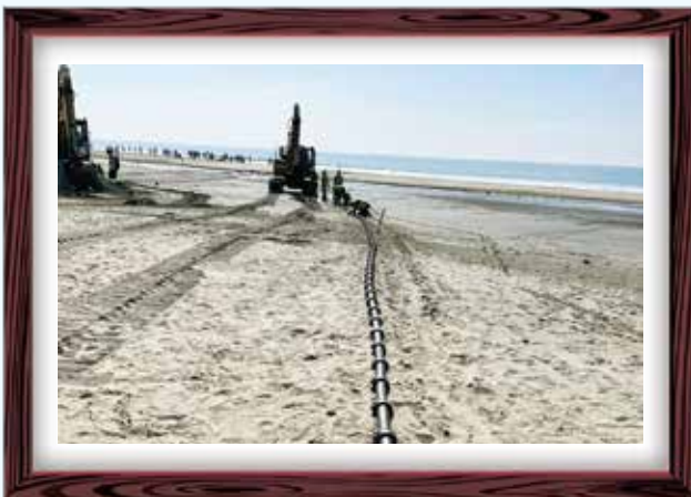
Installation of Cox's bazar branch of SMW-6 submarine cable system at sea beach.
