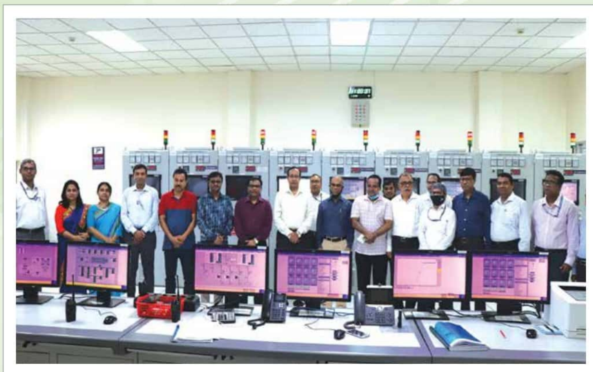
Hon'ble Secretary, Power Division, Chariman, BRPL & BPDB along with Board Directors and High Officials Visit Kodda 150 MW Dual Fuel Power Plant
