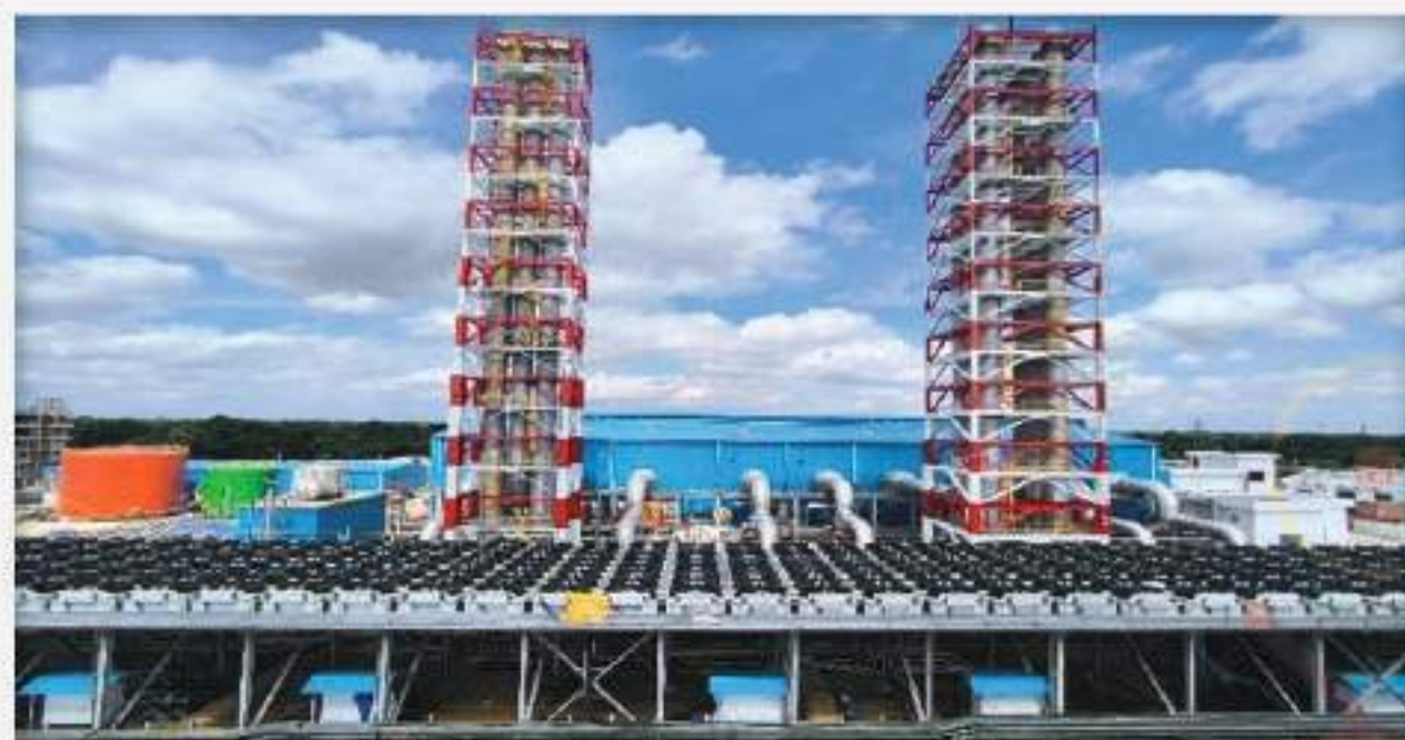
Sreepur 150 (±10%) MW HFO Based Power Plant Project
