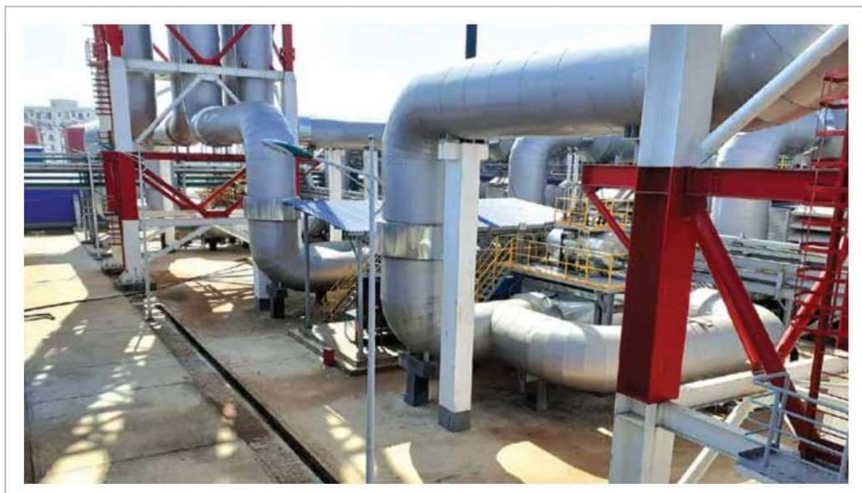
Mirsarai 150 ( \pm 10\% ) MW Dual Fuel (Gas/HFO) Power Plant Project EGB & Auxiliary Boiler Area
