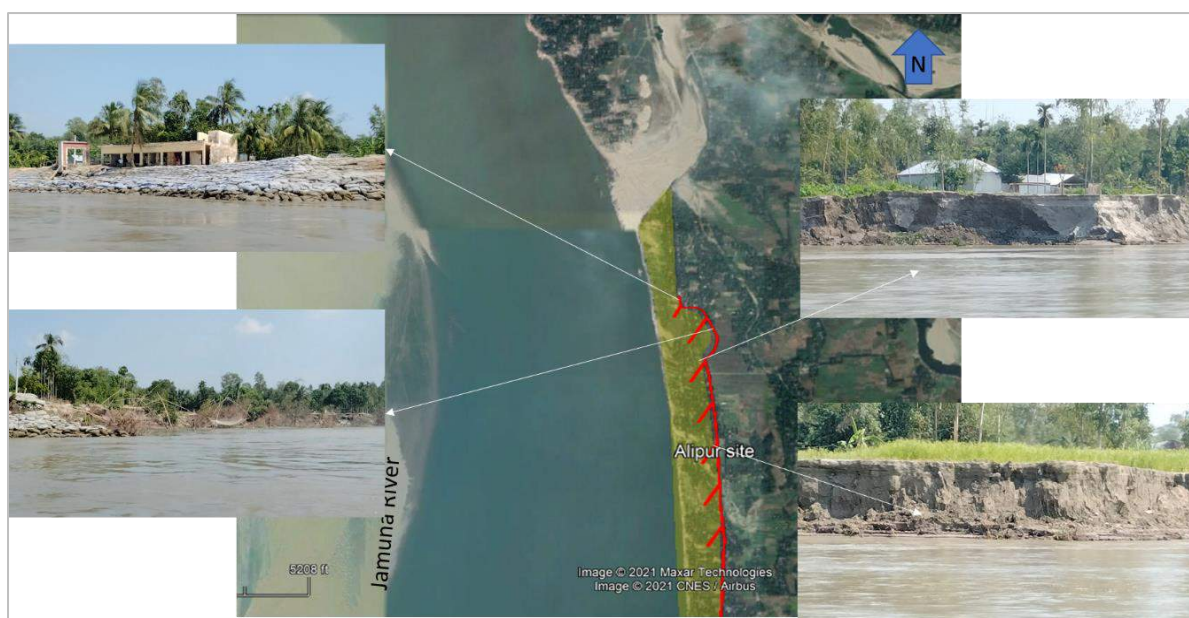
Figure 3.7: Riverbank Erosion along the Kalihati Site
