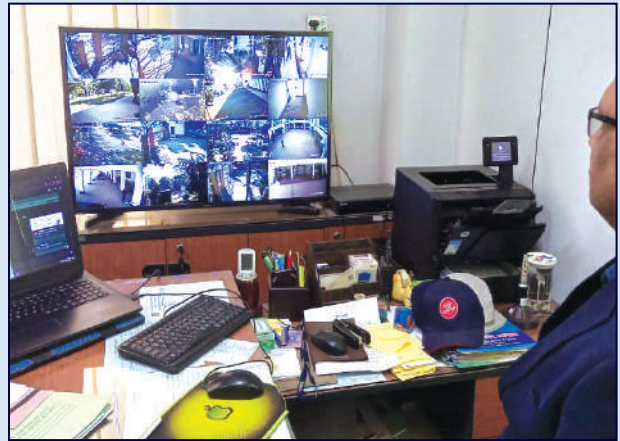
Security monitoring through installed IP cameras at company's head office.
