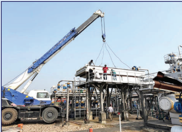
Replacement of a new tube-bundle of process plant's air cooler along with gas flow-line modification at Titas Location-I.
