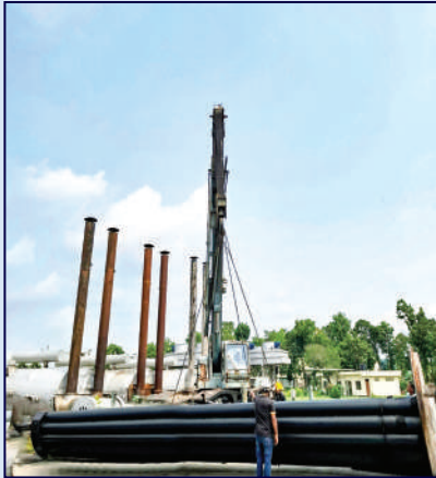
Leakage of gas tube of the oil bath heater-'D' of Bakhrabad field was repaired by company's own manpower.
