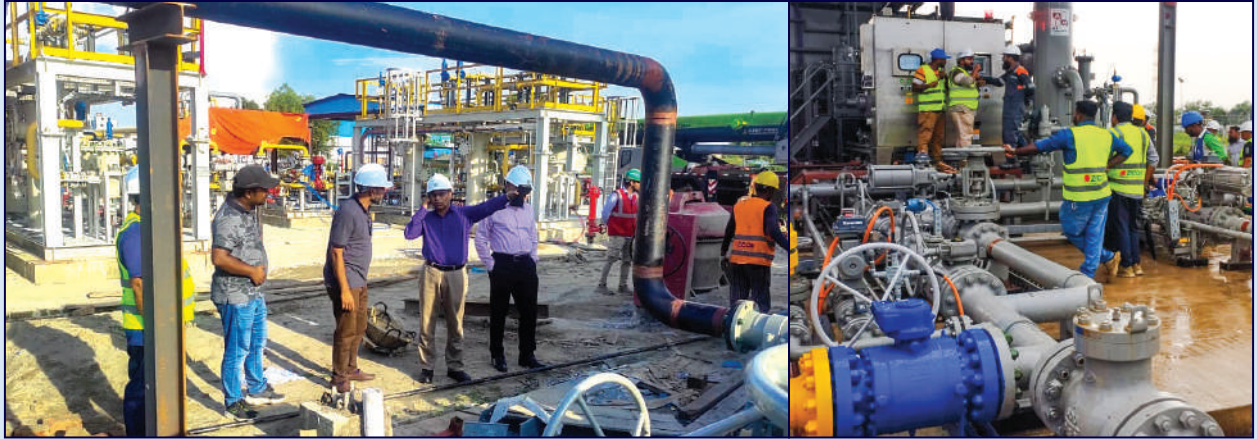
Installation work of wellhead compressors at Titas-G location. Mentionable, 06 wellhead compressors installed at Titas-E & G (3 nos. each) have added nearly 23 MMscfd gas to the national grid.
