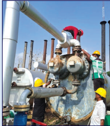
Leakage in fire tube of oil bath heater-'B' of Bakhrabad field repaired by company's own manpower.
