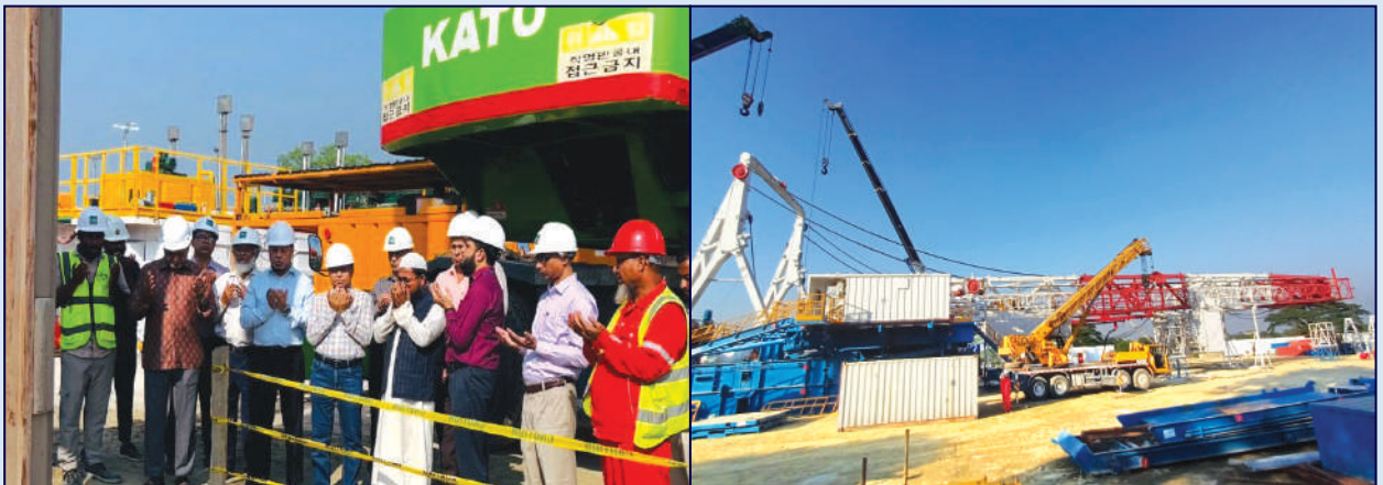
Prayer before 30-inch conductor casing running and the rig-up works aiming to begin drilling of Titas-28, 29 & 30 wells at Location-C under a project.
