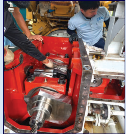
Major overhauling work of post 53,000 running-hours of 03 booster compressors installed at Bakhrabad field.
