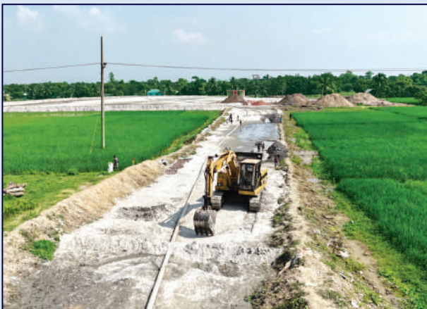
Land development works in the requisitioned area for drilling a deep well (Titas-31).
