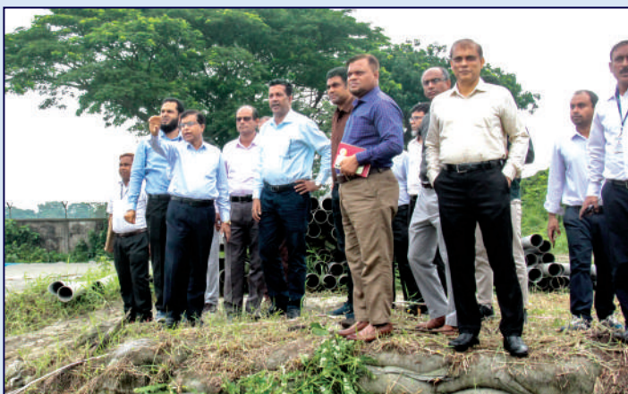
Mr. A K M Mizanur Rahman, Director (Finance), Petrobangla, visiting Titas-28, 29, 30 wells' drilling project site.
