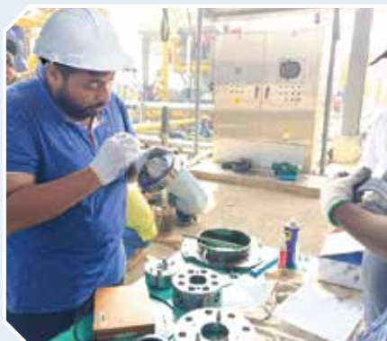
Maintenance works of newly installed compressors at Titas Gas Field are being executed by BGFCL's own manpower.
