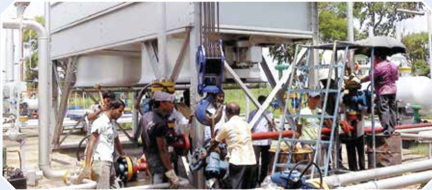
Maintenance work for the cooler of gas process plant at Titas Gas Field.
