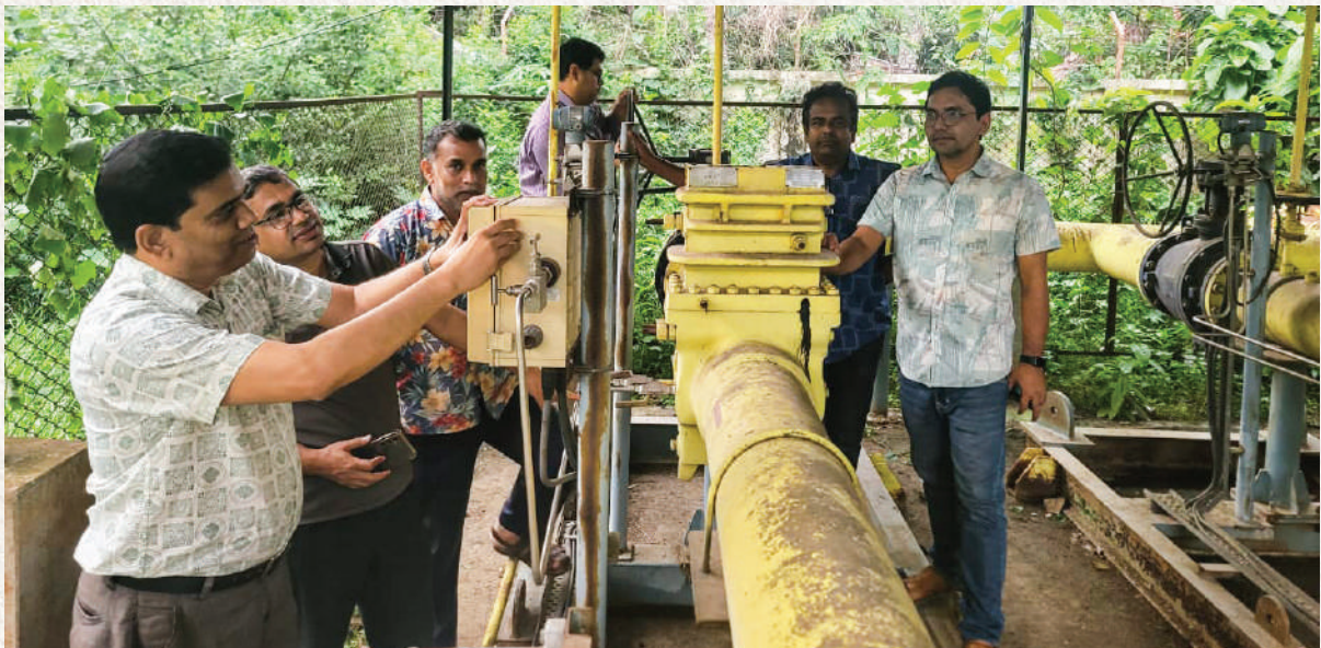
Flow computer of orifice meter is checking and monitoring at Chadpur Power Station
