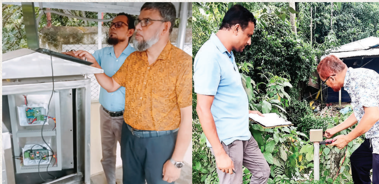
◆ CP station (Transformer Rectifier) online monitoring and Pipe to Soil Potential (PSP) data testing
