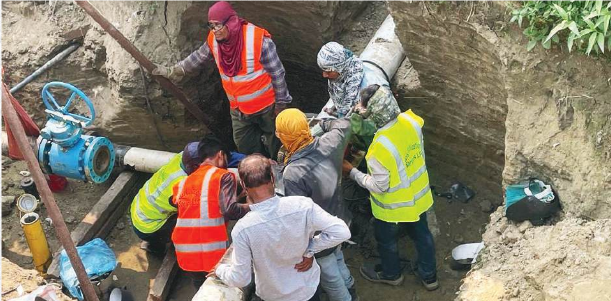
Hook-up activities going on at 6" Transmission line for supply of gas at Ellite Hi-Tech Industry
