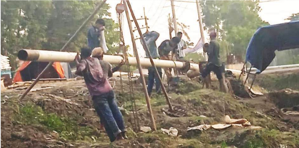
Shifting of gas pipeline for the project of "Upgradation of Feni-Noakhali National Highway From Begumganj to Sonapur to 4 lane"
