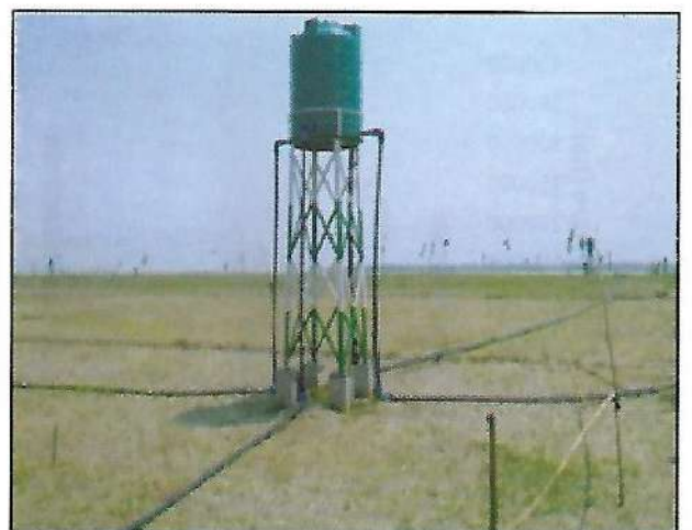
Figure 34: Portable Distribution System in Char Area, Lalmonirhat.
