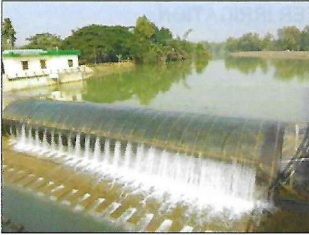
Figure 21: Chellakhali Rubber Dam, Nalitabari, Sherpur.
