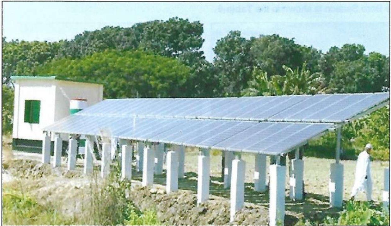
Figure 27: 0.5 Cusec Solar LLP at Dhamrai Upazila, Dhaka.
