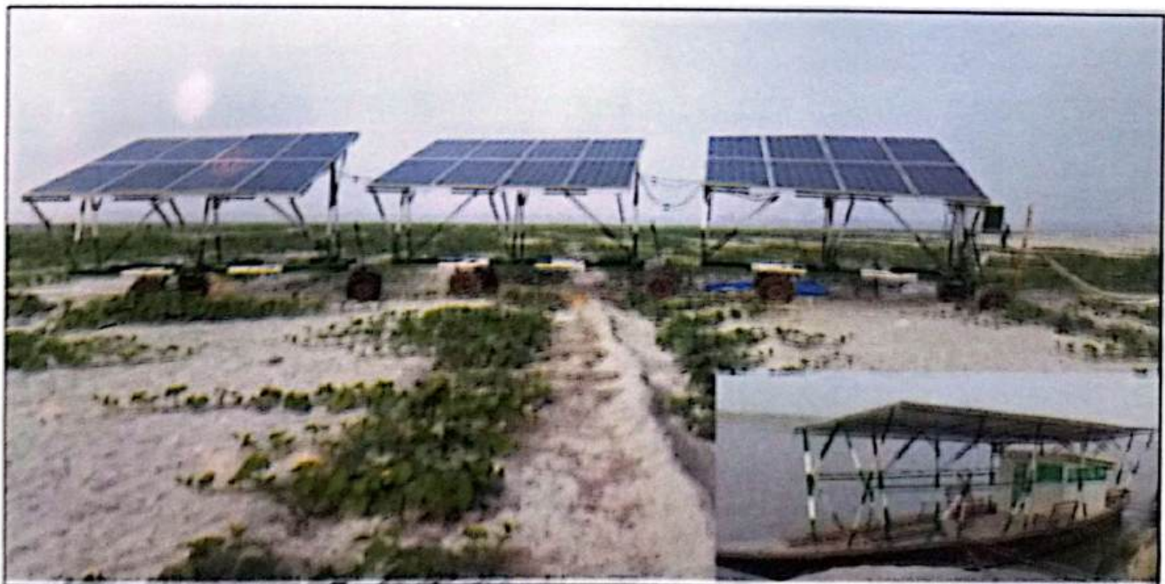
Figure 27: Portable Solar LLP at Char Area, Rangpur.
