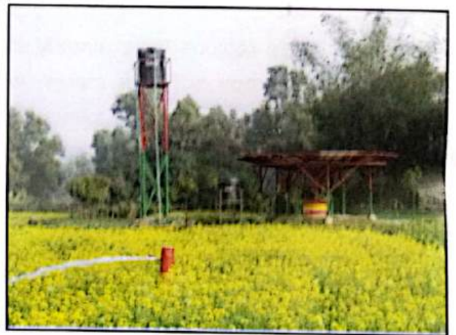
Figure 8: BMDA Solar Energised Dug Well in Shapahar Upazila, Naogaon
