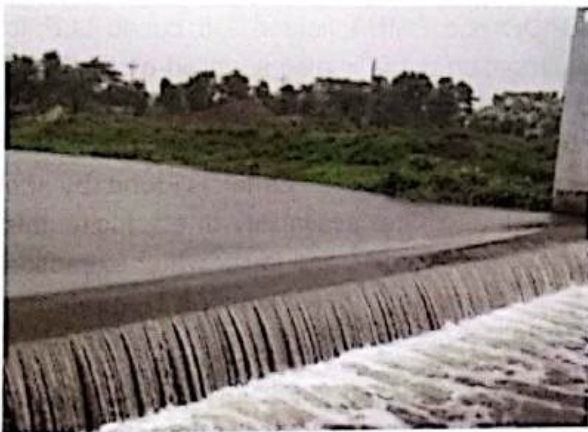
Figure 32: Submerged Weir at Ashuganj-Palash Agro Irrigation Project by BADC
