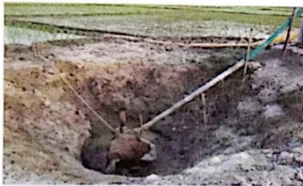
Figure 17: Shallow Tubewell (pit) at Baghmara Upazila, Rajshahi
