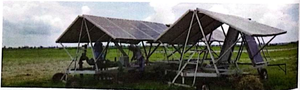
Figure 19: Portable Solar system for STW operated by BADC at Kaunia Upazila, Rangpur
