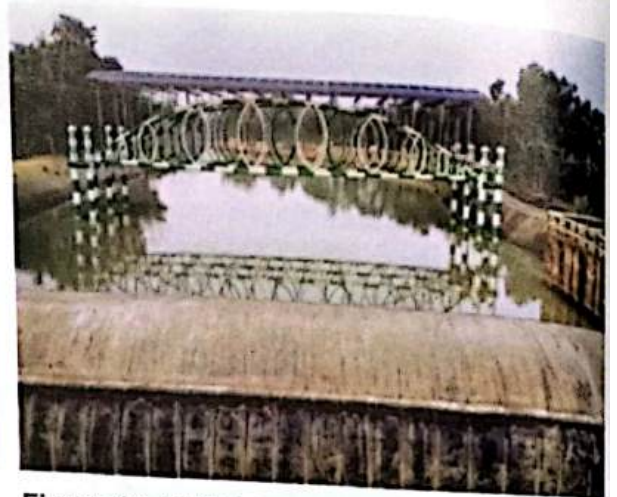
Figure 46: Chillakhali Nodi Rubber Dam at Nalitabari, Sharpur by BADC
