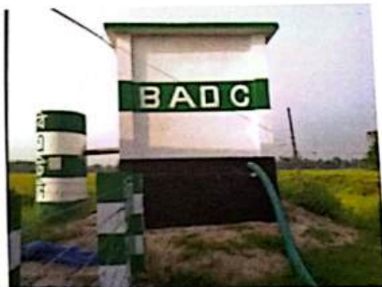
Figure 36: LLP with Buried Pipe, Nangalkot Upazila, Cumilla by BADC
