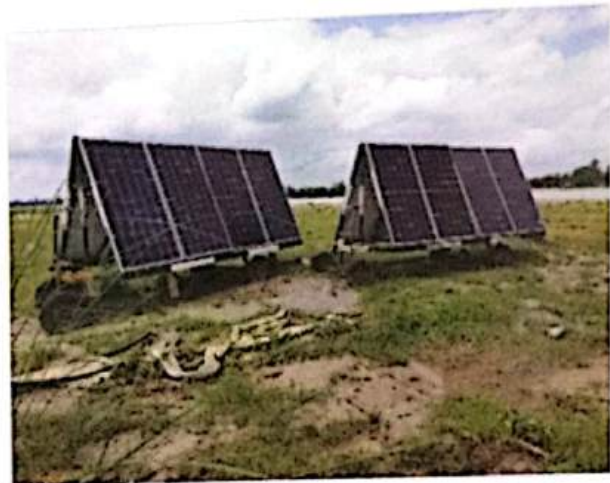
Figure 43: Portable Solar Irrigation System by BADC at Char area Rangpur
