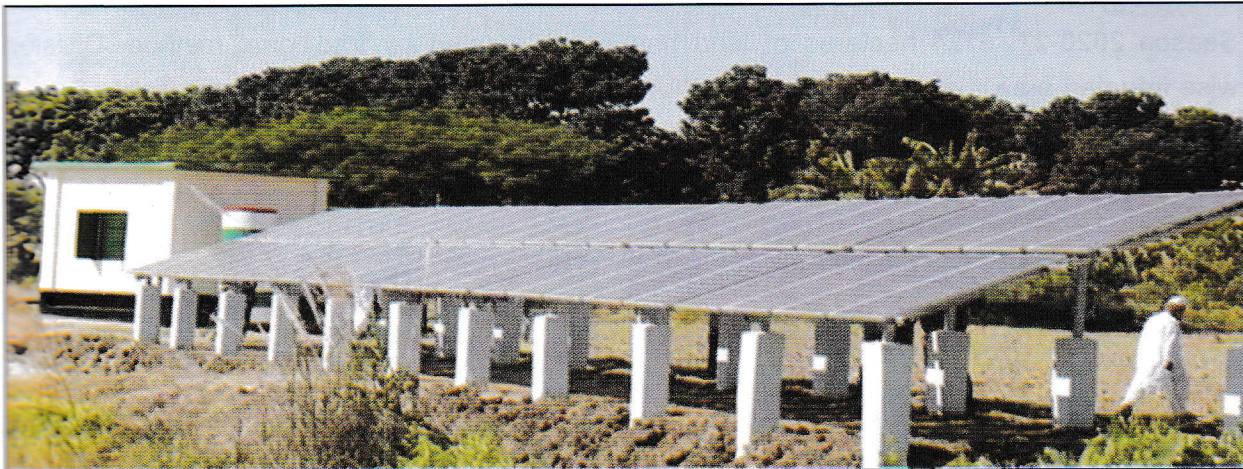
Figure 27: 0.5 Cusec capacities Solar LLP in Dhamrai Upazila, Dhaka.
