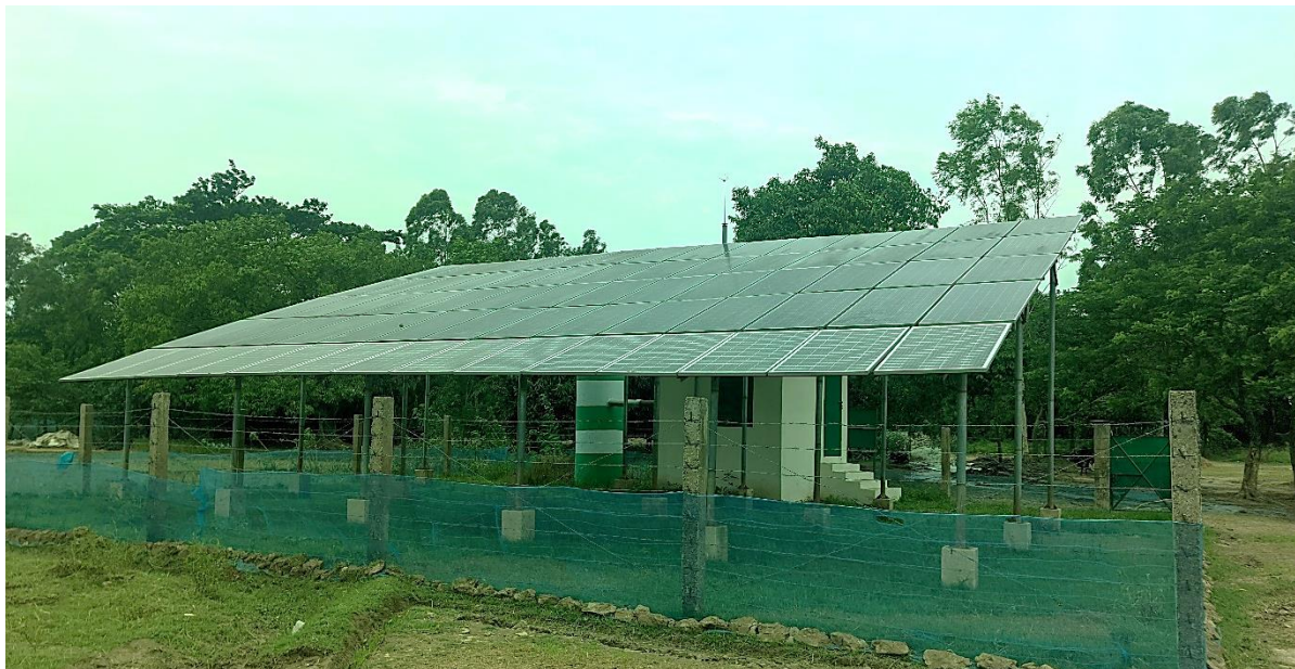
Figure 5.36: BADC Solar Deep Tubewell at Derai Upazila, Sunamganj
