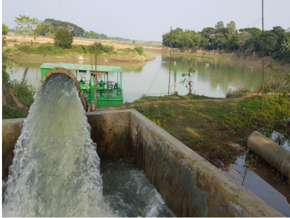
Figure 5.13: 25 Cusec Floating Pump at Atpara Upazila, Netrokona by BADC
