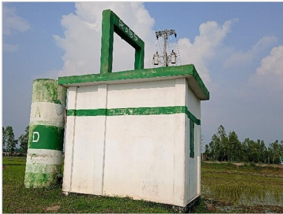
Figure 5.34: BADC Deep Tubewell at Lakhai Upazila, Habiganj
