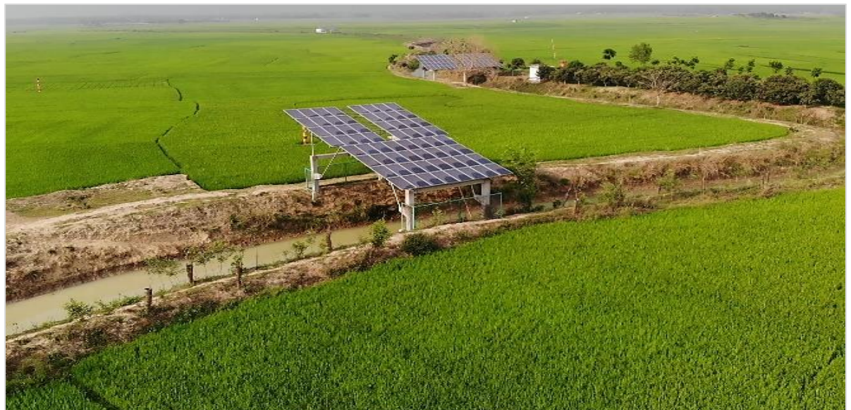
Figure 5.18: Solar LLP at Rajshahi by BMDA
