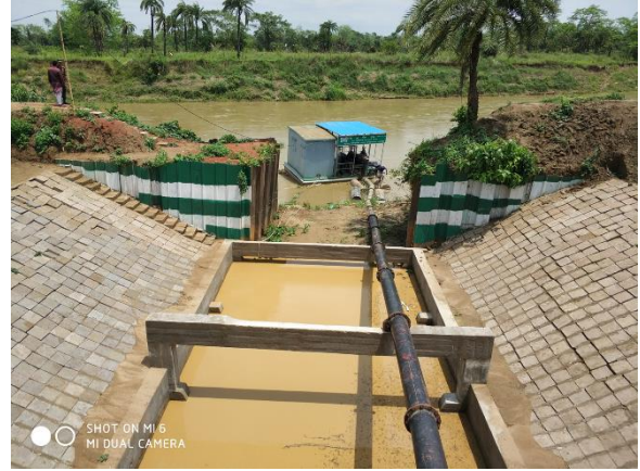
Figure 5.14: 10 Cusec Floating Pump at Adarsha Sadar Upazila, Cumilla by BADC
