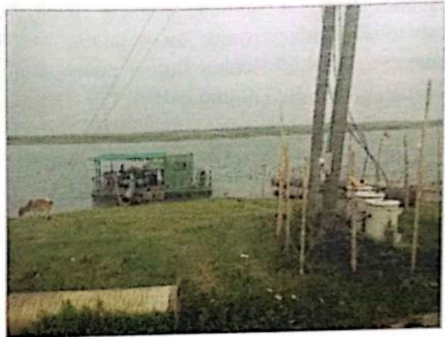
Figure 40: 12.5 Cusec Floating Pump, Netrokona
