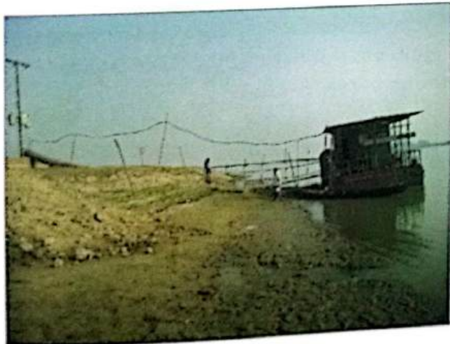
Figure 41: 12.5 Cusec Floating Pump, Sunamganj
