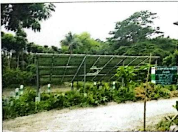
Figure 37: 0.5 Cusec Solar LLP at Kolaroa Upazila, Satkhira
