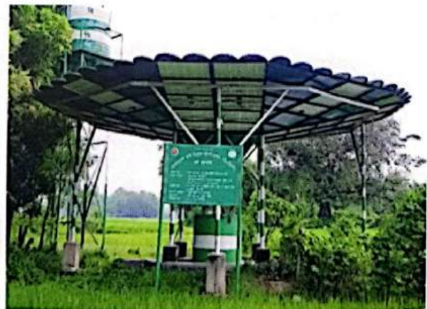
Figure 23: BADC Solar operated Dug well in Porshuram Upazila, Feni District.
