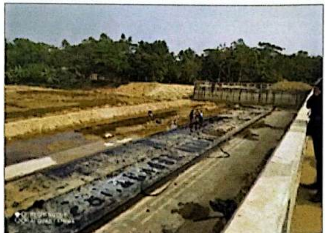
Figure 46: Netai River Rubber Dam at Dhobaura Upazila, Mymensingh by LGED.
