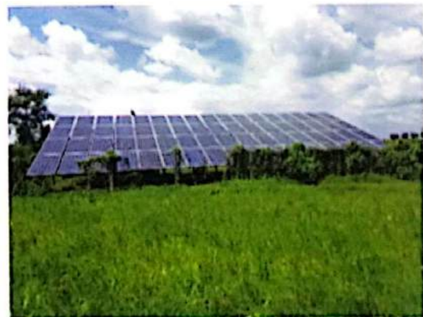
Figure 14: Solar DTW at Bochaganj Upazila, Dinajpur
