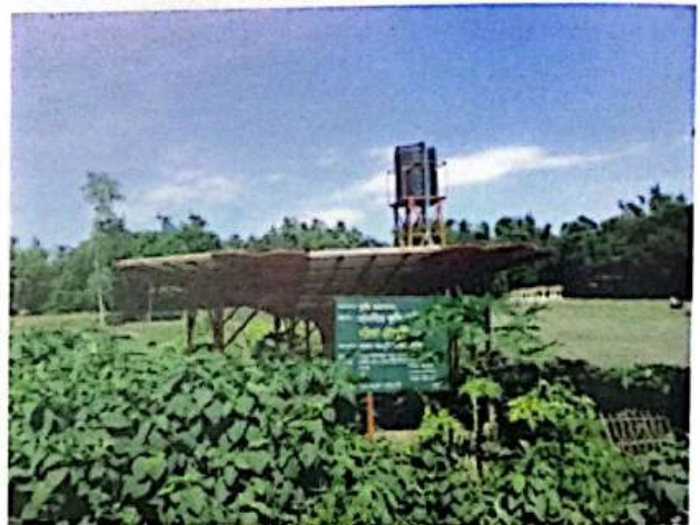
Figure 21: BMDA Solar operated Dug well in Saidpur Upazila, Nilphamari District.
