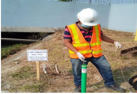
Ground water level measuring
