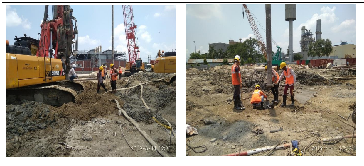
Figure 4.8: At the Construction Works, Workers were Found with Proper Apron, Helmet and Hand Gloves etc.
