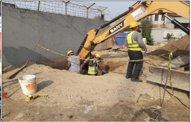
Hazardous area kept isolated
