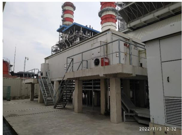
Power control center
