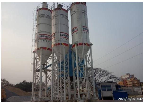
Fig: Batching plant
