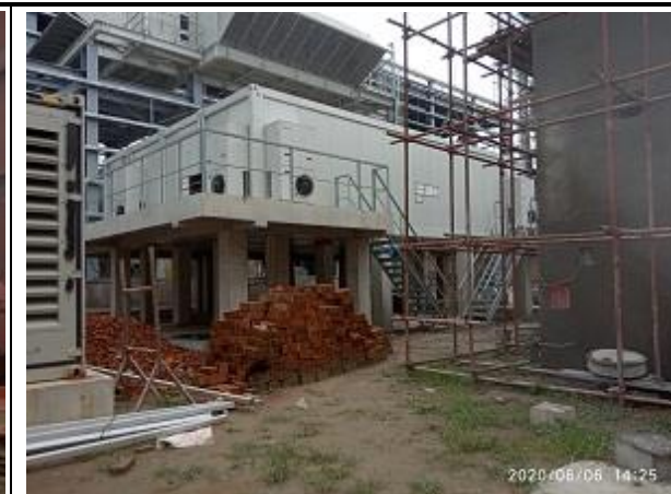
Fig.: Power Control Centre
