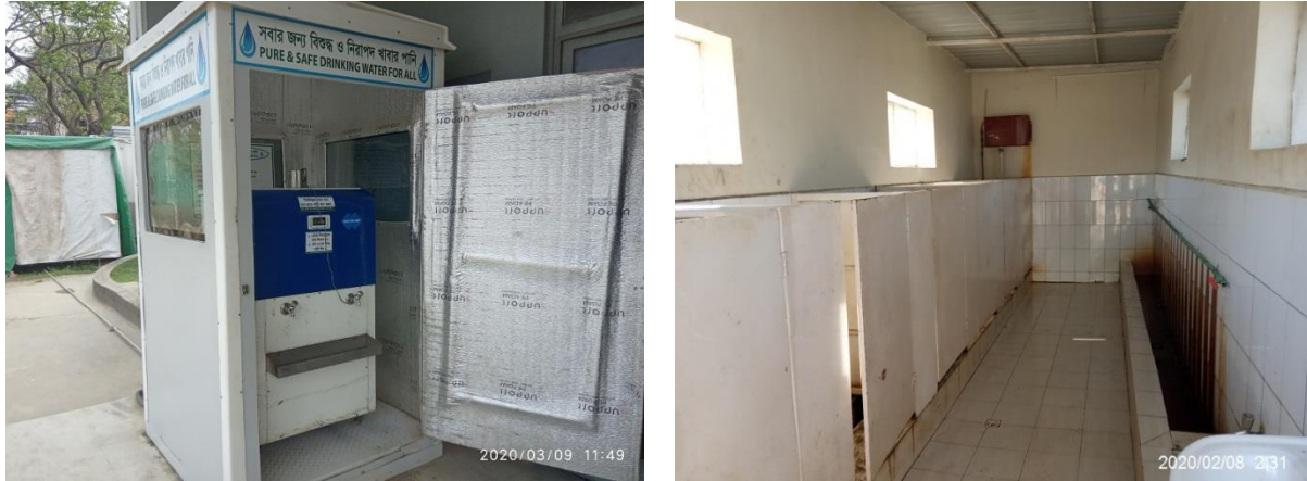
Figure -13: Pure Drinking Water & Sanitation facility to workers
