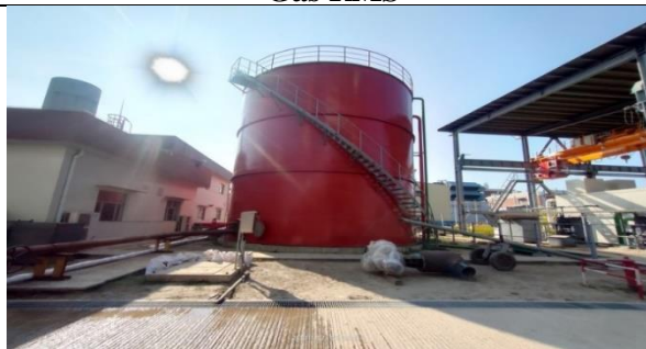
Service and Fire Water Tank
