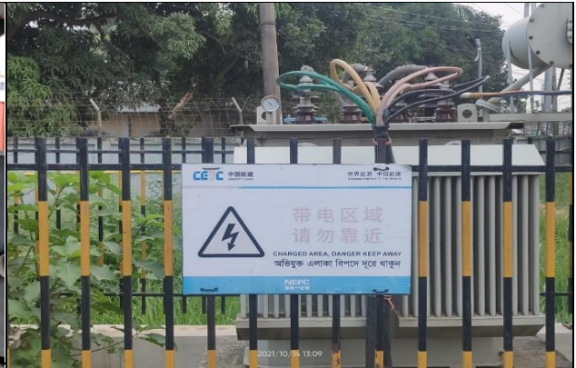
Hazardous area kept isolated
