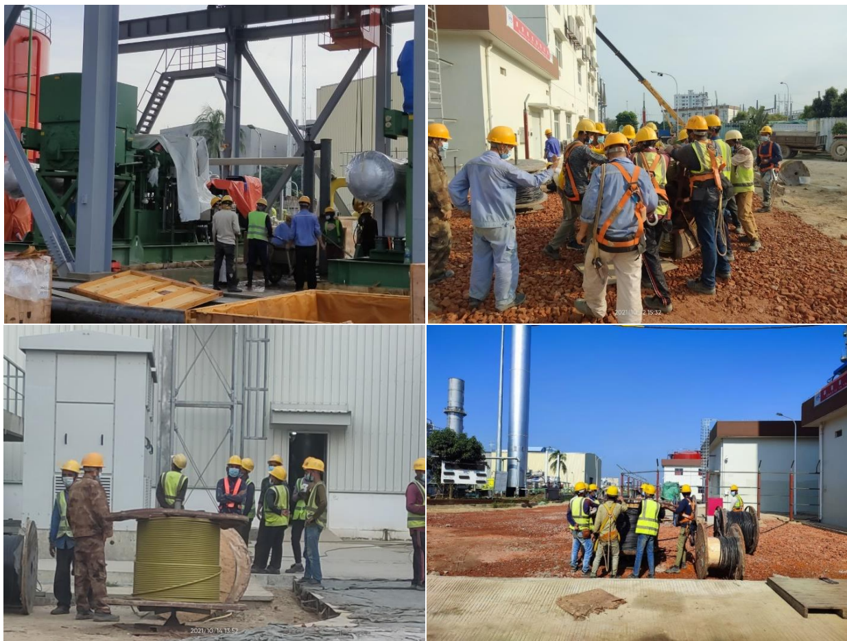
Figure 5: Use of Proper PPEs
