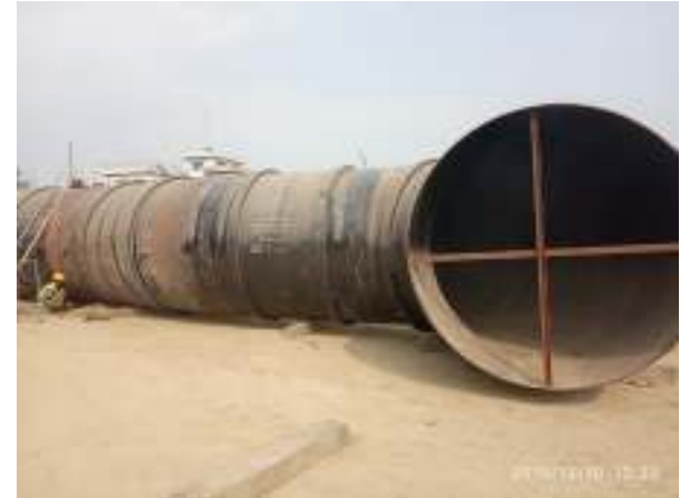
Water Discharge Pipe
