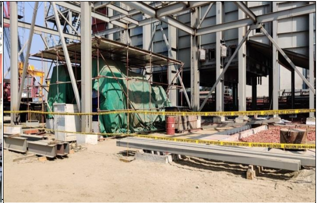
Hazardous area kept isolated
