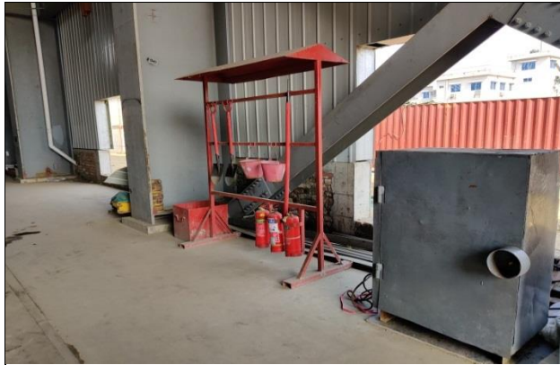
On-site Firefighting Appliances
