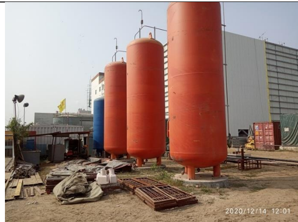
Hydrogen Storage Tank
