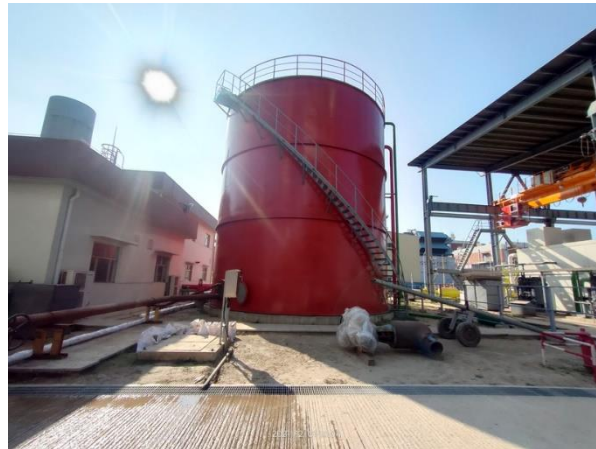
Fig. 1.2.5: Service and Fire Water Tank
