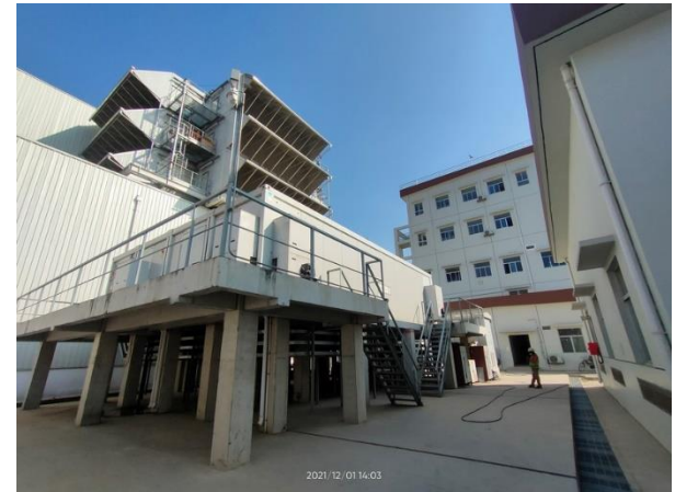
Fig. 1.2.6: Power Control Center
