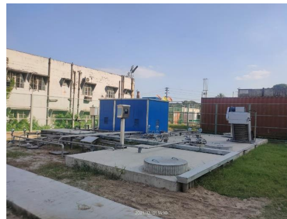
Fig. 1.2.9: Sewage treatment station
