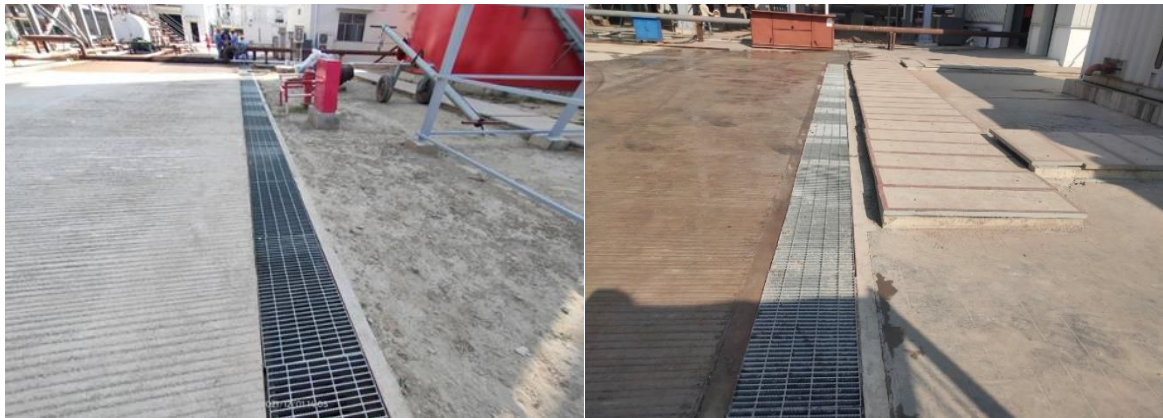
Figure 20: Photograph of Site Drainage
