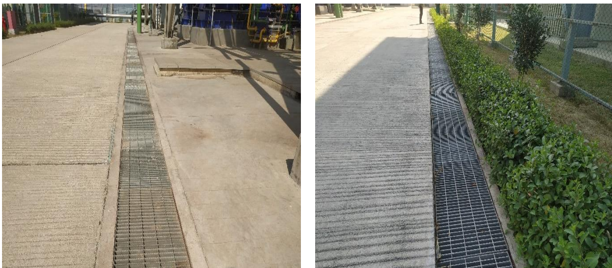
Figure 13: Photograph of Site Drainage
