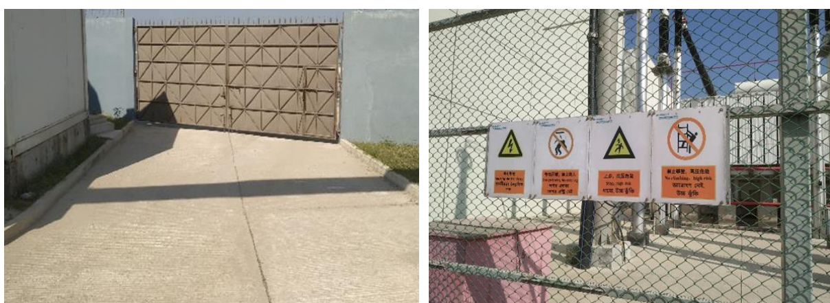
Figure 7: Present Boundary Wall Condition & Warning Signage at the Plant Site
