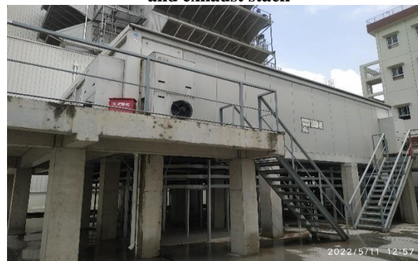
Fig. 1.2.6: Power control center
