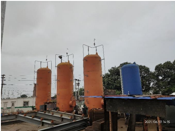
Hydrogen Gas Receiver
