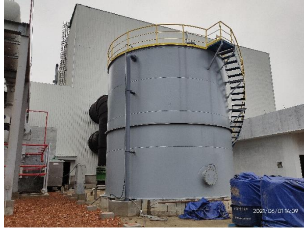
DIL Water tank
