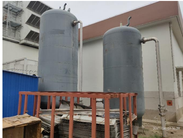
Air Storage tank
