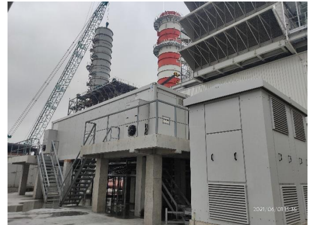
Power Control Center
