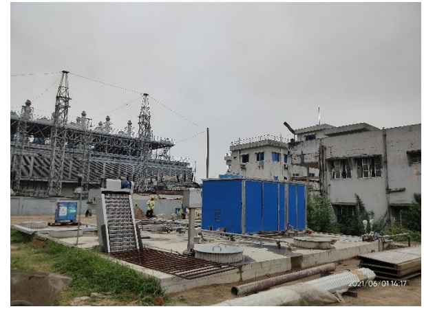
Sewage treatment station
