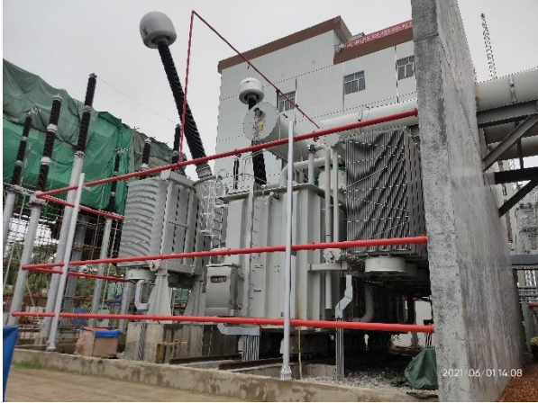
Generator Step up transformer
