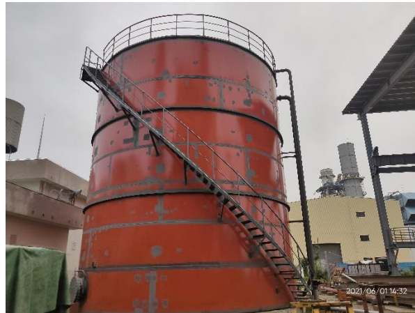
Service and Fire Water Tank
