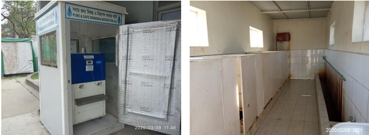
Figure -18: Pure Drinking Water & Sanitation facility to workers
