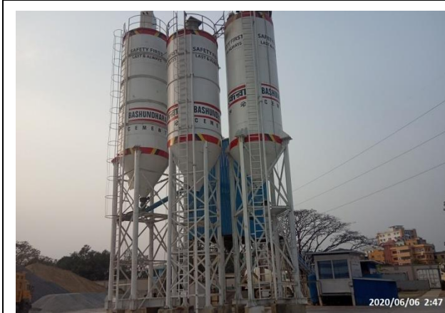
Fig: Batching plant
