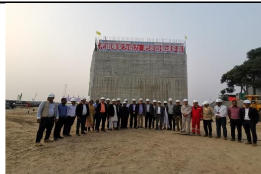
Inauguration of CW pump house by Chairman of APSCl
