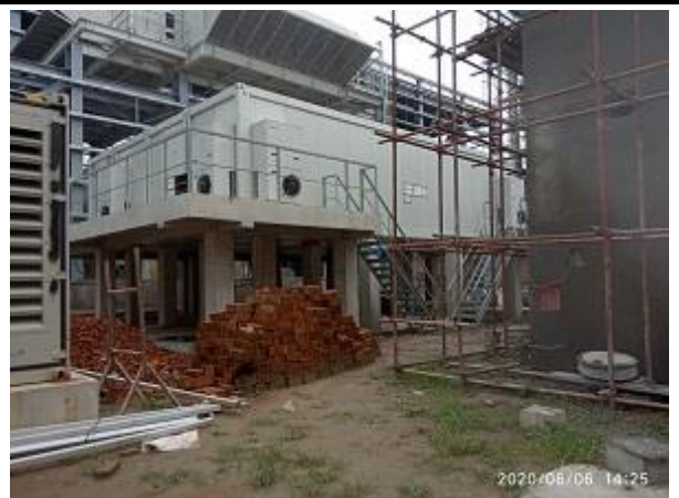
Fig.: Power Control Centre
