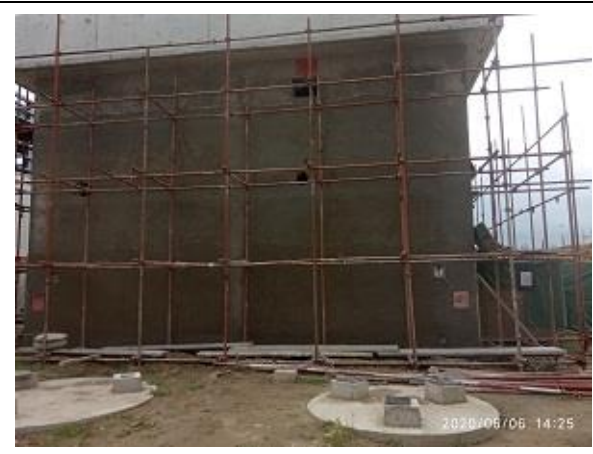
Fig: Construction of oily waste water treatment station and service fire water tank
