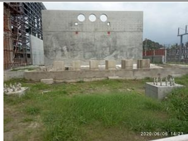
Fig: Generator Setup transformer location
